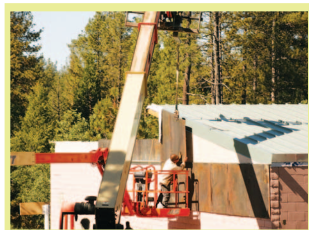
Construction of the new Idyllwild Library continues with the placement of steel frames along the building's north side.
