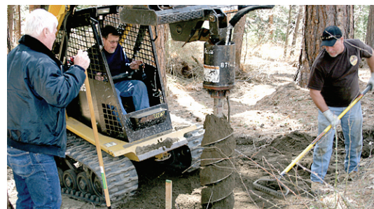
From left, Rotary president Danny Richardson , Rick Foster and Dan Slattery , co-owner of Honey Buns and Joe , all volunteered their time at the future Idyllwild Community Center property last weekend. The trio, with the use of Foster's Compact Track Vehicle, dug post holes that will eventually be used to anchor exercise equipment.
