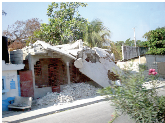
A photo of a collapsed building in Haiti following the Jan. 12 earthquake taken during local Susan Swanson's volunteer mission to Cap Haitien, Haiti.
