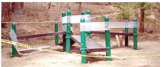
Station #2, the toe reach station, on the new fitness par course on the Idyllwild Community Center property on Highway 243, is nearing completion. The project is being built by volunteers.
