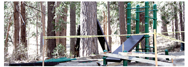
As of Friday, sections of the new par course were not finished, but well on the way. Yellow caution tape was wrapped around sections that were not completed to keep people off of the equipment.
