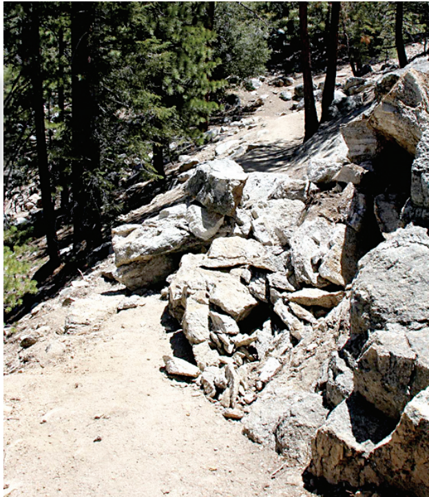
This rockslide (above), about 1/2 mile from the top of the Ernie Maxwell Scenic Trail, occurred last week. Bob Haine and his wife took this photo and said, "In spite of the necessary detour around or over the rocks, there were quite a few hikers and their canine companions on the trail."
