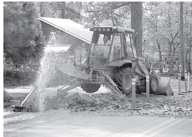
Jim Hamilton , who was an Idyllwild Water District field maintenance worker, digs up a section of Upper Pine Crest to get to a worn connection that had burst in January 1993.
