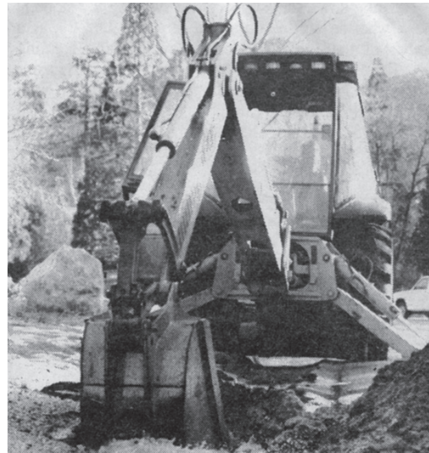
In January 1991, Idyllwild Water District field personnel, while trying to fix a leaky line on Ridgeview Drive, ruptured it further because the line was inaccurately marked. It was repaired soon enough to avoid any drop in the district's supply. FILE PHOTO
