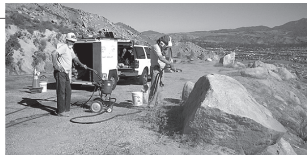
Members of the Mountain Community Patrol removing graffiti from a rock on Highway 243.
