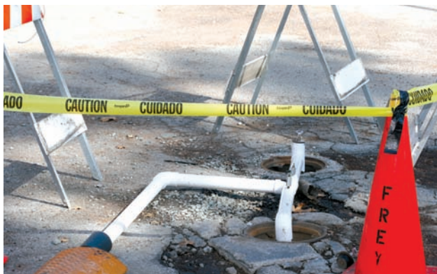
A soil vapor extraction of volatile hydrocarbons is being conducted at the Pine Cove Market, where the chemicals had escaped tanks and leaked into the subsurface years ago. This is part of an ongoing effort to clean the area.
