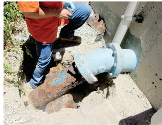
The hole in this portion of the Idyllwild Water District's sewer pipe demonstrates the need for major repair work and pipeline replacement. PHOTO COURTESY OF TOM LYNCH, IDYLLWILD WATER DISTRICT
