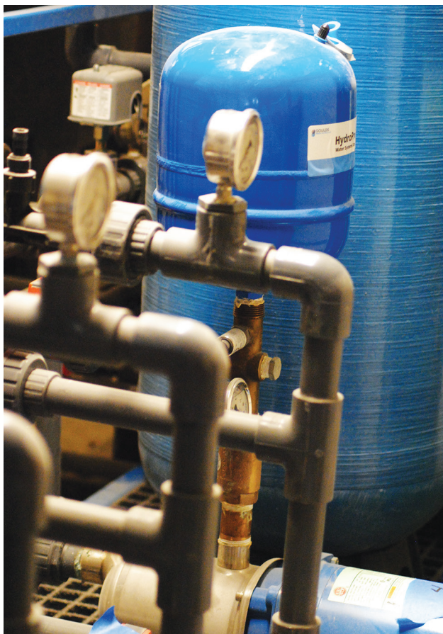
Part of the piping to help reclaim the water to be used at the coming Idyllwild Brewpub. PHOTO BY JP CRUMRINE
