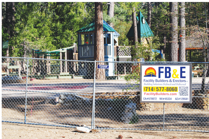
Left, construction is beginning at the Idyllwild Community Center site. Grading and road-work are the first phases of work. PHOTO BY JP CRUMRINE
