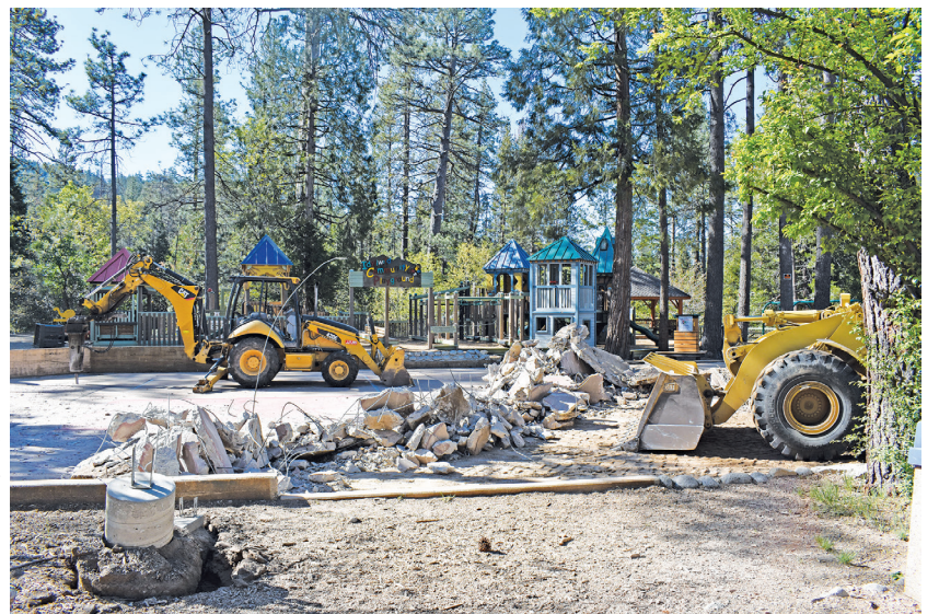
Right, work to demolish the tennis court at the site of the future Idyllwild Community Center was in progress Tuesday morning. PHOTO BY HALIE WILSON
