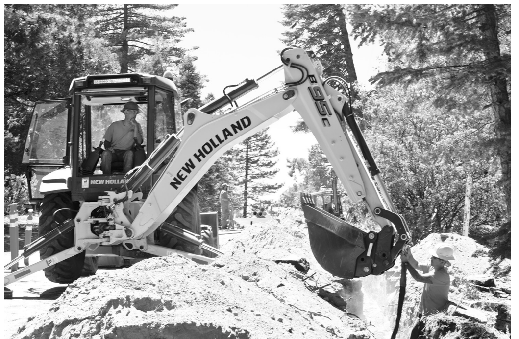
In the summer, the Pine Cove Water District crew replaces and installs new pipelines. Here they are laying a new 8-inch water main along Pine Ridge as part of the South Central Pipeline Installation Project in Pine Cove. The district's goal for this summer is to lay 2,000 feet of new mains and fire hydrants. PHOTO BY STEVEN KING
