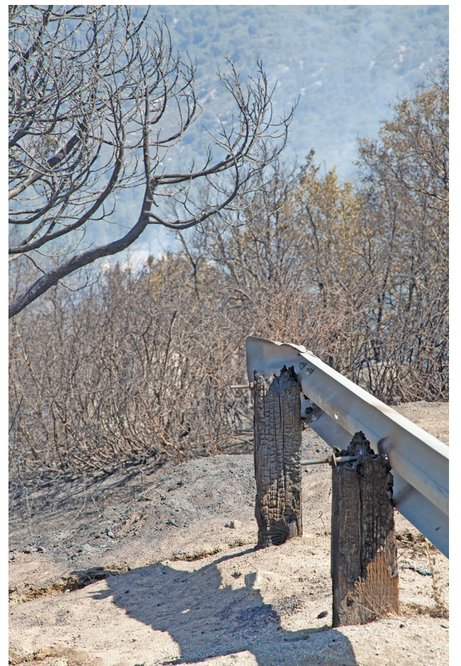
The wooden guard rail supports are burned. One of the reasons Caltrans has much work to do before re-opening Highways 74 and 243. PHOTO BY STEVEN KING
