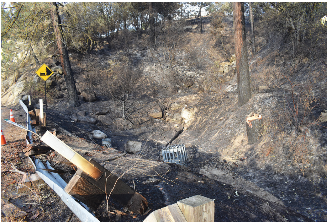
The guardrail and a large culvert on Highway 74 between McGaugh Road and McCall Park Road were severely damaged as the Cranston Fire ripped through the canyon below, eventually destroying a home at the top of the hill. PHOTO BY HALIE WILSON
