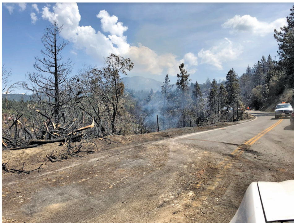
Damage from the fire and heavy equipment can be seen along Highway 243 in Mountain Center, where Caltrans crews were hard at work doing repairs. PHOTO BY CALTRANS SUPERINTENDENT JOHN HUBBS
