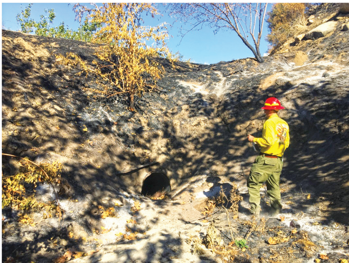
After the Cranston Fire, a member of the Burned Area Emergency Team examines the potential damage to a culvert near a Forest Service road.
