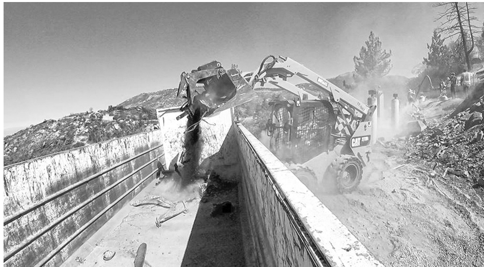
Riverside County workers clean up debris resulting from the Cranston Fire. PHOTO COURTESY RIVERSIDE COUNTY DEPARTMENT OF WASTE RESOURCES
