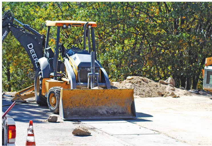
The Idyllwild Water District recommended that the fire suppression water pipeline for the Idyllwild Community Center connect to the fire pipeline in Strawberry Plaza. This construction, in front of Fairway Market, started last week. PHOTO BY JP CRUMRINE
