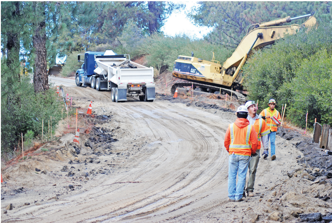
Caltrans is repairing a culvert under Highway 243. Since the work requires removal of the highway surface to replace the old with a new culvert, the highway is closed in both directions at that area. The project is just north of Lake Fulmor. PHOTO BY JP CRUMRINE
