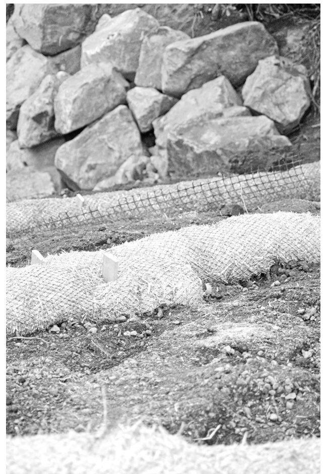
Highway 243 was closed so that a culvert could be replaced. This view is from the highway looking down the slope to the culvert opening.
