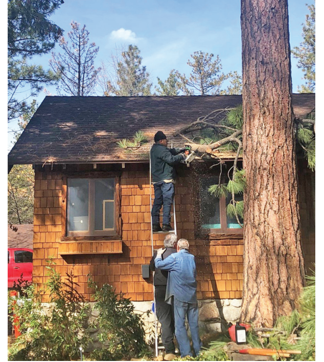
The storms last week caused some damage to the Idyllwild Area Historical Society (IAHS) building. A tree branch fell off and went through the roof like a spear. When Docent Nancy Borchers walked in to open the building for visitors on Friday, Dec. 6, she found the tree branch in the building. Within a very short period of time, Manuel Guzman (on ladder), Richard Levitski , Larry Robinson , and Tom and Marlene Pierce were there to help get the branch out of the roof. George Groty got a tarp to place over the opening in the roof for the time being. IAHS does own the building, thanks to the help of former Riverside County Supervisor Kay Cenicerros .
